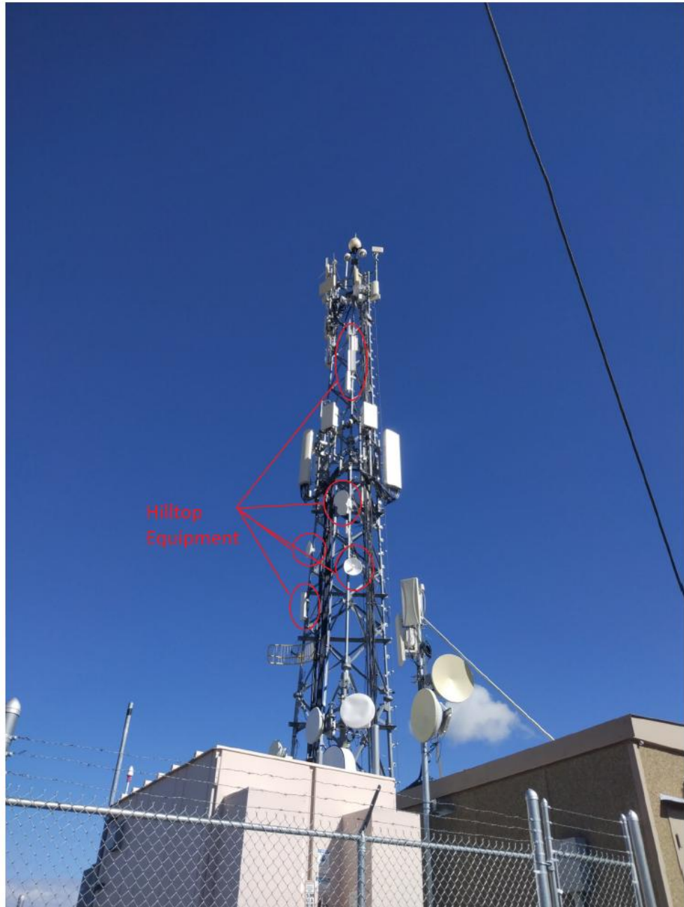
View of Hilltop Broadband Equipment on Tower (1 of 2)
