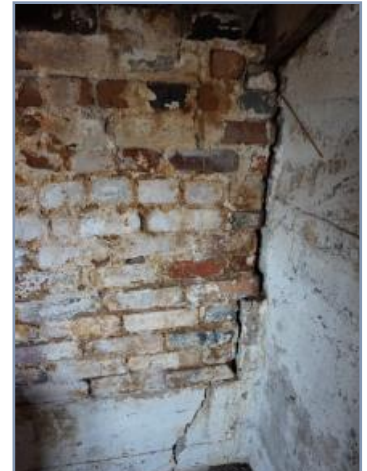
Crack in masonry wall
